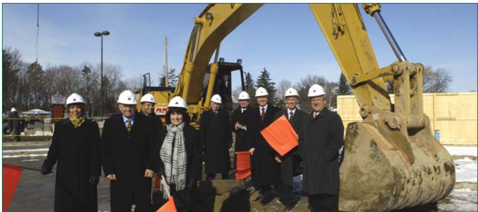
Flagging the Backhoe Operator to begin the Ground Breaking are (left to right):
